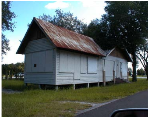
Major deterioration of a single-family residence
