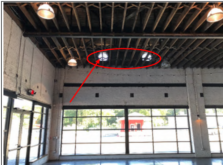
Photo No. 4 Interior view of reflecting the areas where leaks have been identified. Note "vent" features are open to exterior.
